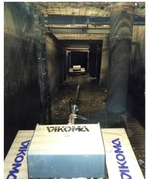
Skimmers in situ in empty sump
